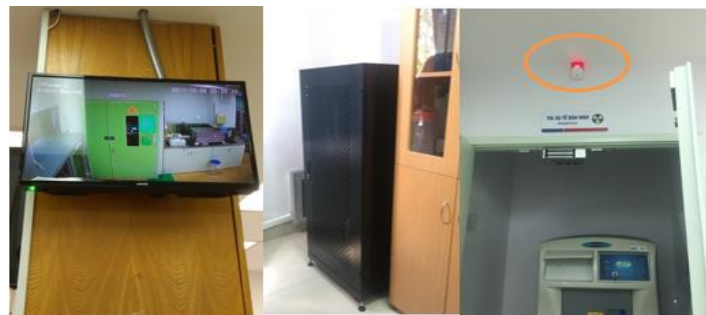
Figure 4: Monitor screen, Central system cabinet, warning light and siren.
